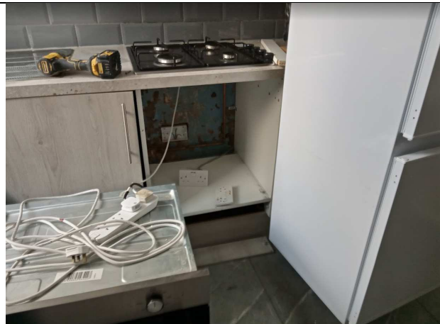
Fig 5. Double socket supplying oven and hob
